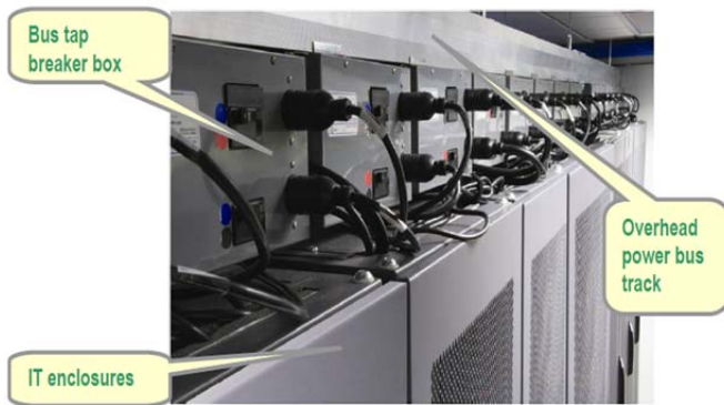
Figure 6. Bus-way to the rack
